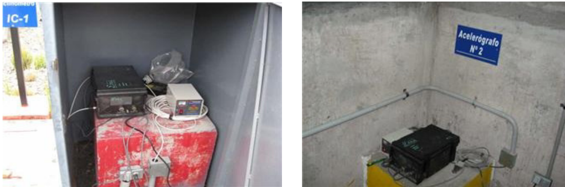
Figure 1. Accelerometers installed in the dam. Left: Accelerometer installed at the crest dam. Right: Accelerometer installed at the bedrock level.
